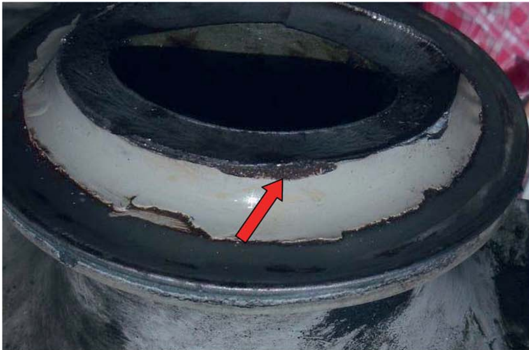
Photo n. 3: presence of uniform corrosion on the external surface, right where the progressive crack initiation.
