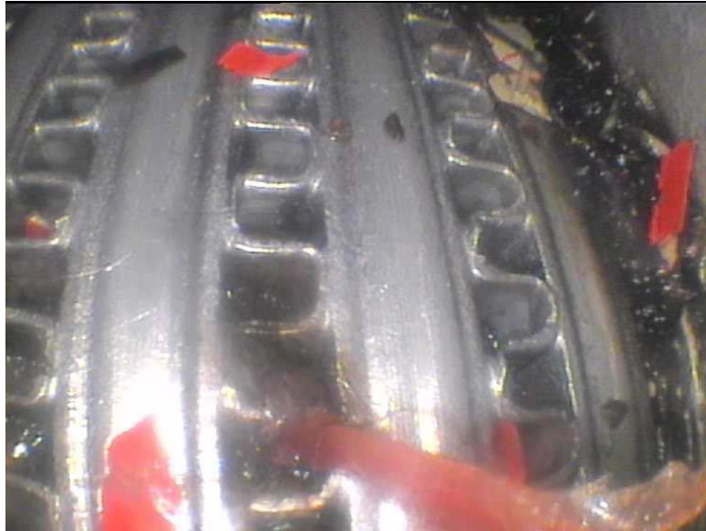
Picture 4: pollution and debris found within the “oil to fuel heater” inlet duct.
